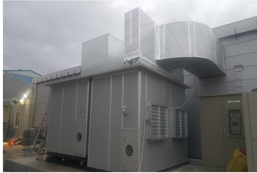
Air Handling Unit(1,644cmm)
