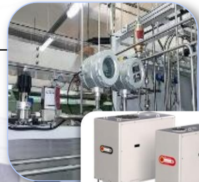
Vacuum and gas piping
